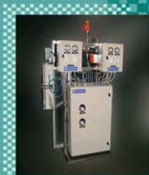
Supply and monitoring block
